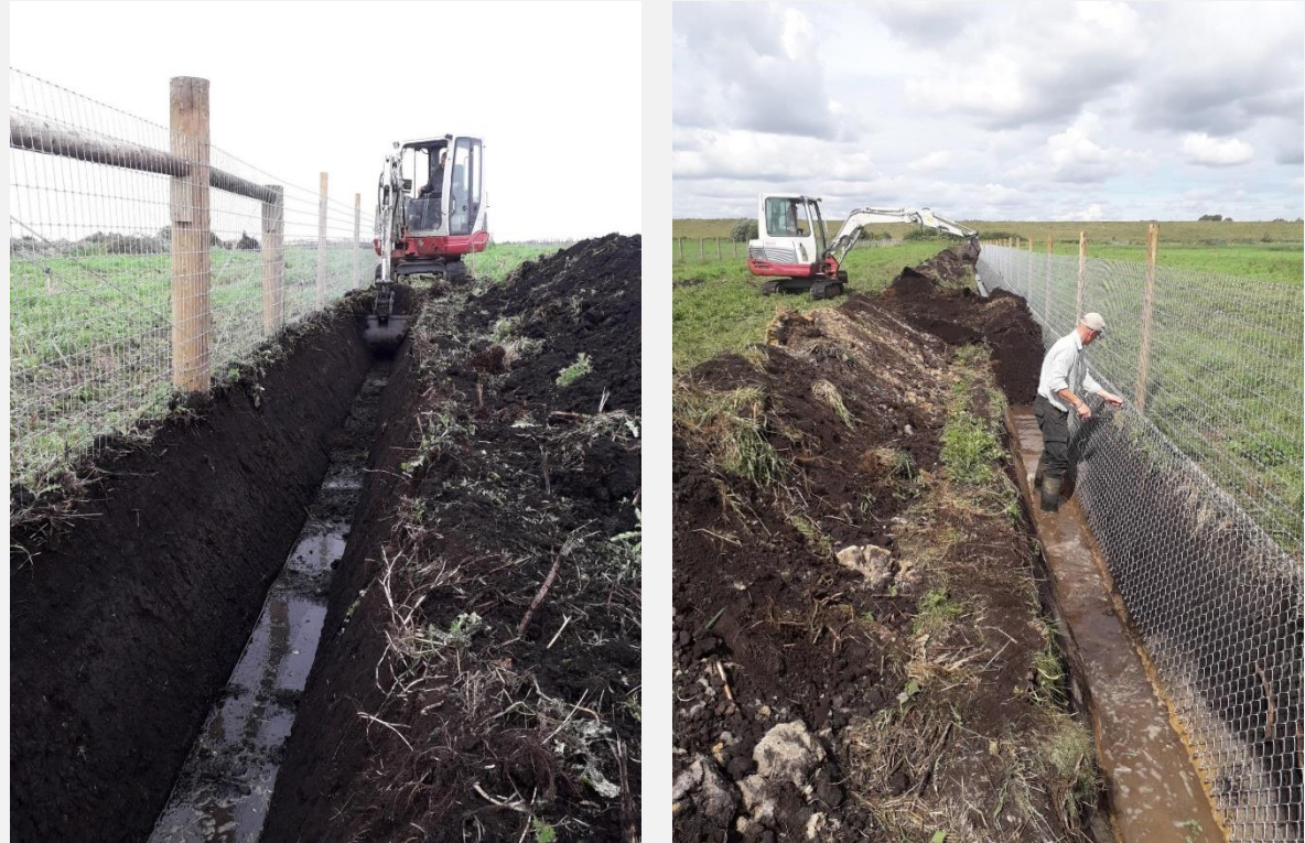
Fig. 17. Installing the underground mesh of a combination fence at Coveney Byall Fen. The left hand photo shows the digging of a trench on the outside of the fence using a 'V' bucket on a mini-digger. Initially, trenches were dug before posts were installed, but the knocking in of the posts in the peaty soil caused too much damage to the trench.
