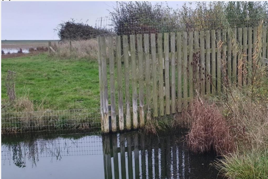
Fig. 30. Two different transitions from barrier fencing around gates over crossings, to in-ditch fencing. (a) Shows a fairly standard wing of a gate at Wallasea Island but which is covered in mesh that has 5cm gaps between its vertical wires, and with mesh also attached to outwardly angled cranks. (b) Wings at Frampton Marsh made of the same half round, smooth pine posts as shown in Fig. 24, which are covered by mesh that has 5 cm gaps between its vertical wires, with this mesh also extending upwards to form a floppy top. In both cases, the outside of the fence is on the near side. Photos by Malcolm Ausden (top) & Toby Collett (bottom).
